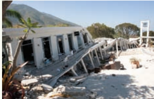
Hotel Montana lies in ruins following the Jan. 12 earthquake. A UMNS photo by Mike DuBose.
